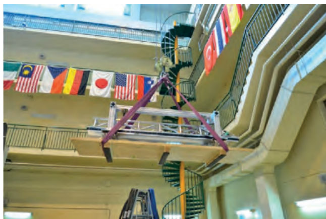
Figure 3: Installation of one of the 16 TOP detector modules in the experimental hall of the Belle II spectrometer. This detector system is being prepared by physicists from Japan, the US, Italy and Slovenia.
