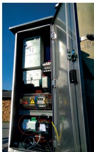
Figure 3: Synchro-phasor measurement unit (red circle) deployed in a real environment on a transformer mast. Developed within FP7 SUNSEED project.
