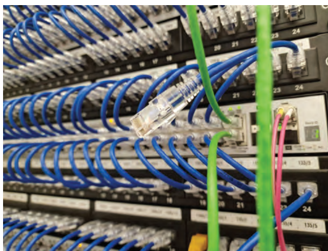
Figure 1: New network cabinets at our new locations
