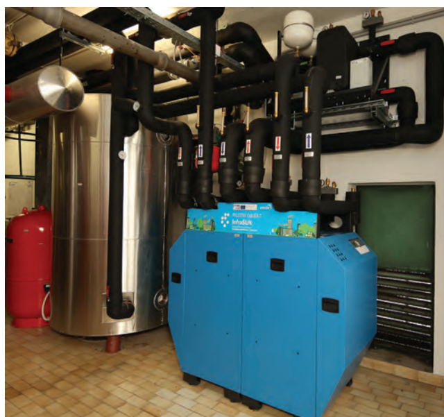
Figure 4: Installation with the adsorption chillers and heat storage (photo: M. Smerke)
