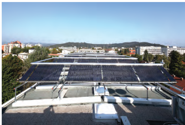
Figure 3: A view to the solar thermal collectors filed ('roll-bond' type) at the JSI headquarters in Ljubljana (photo: M. Smerke)
