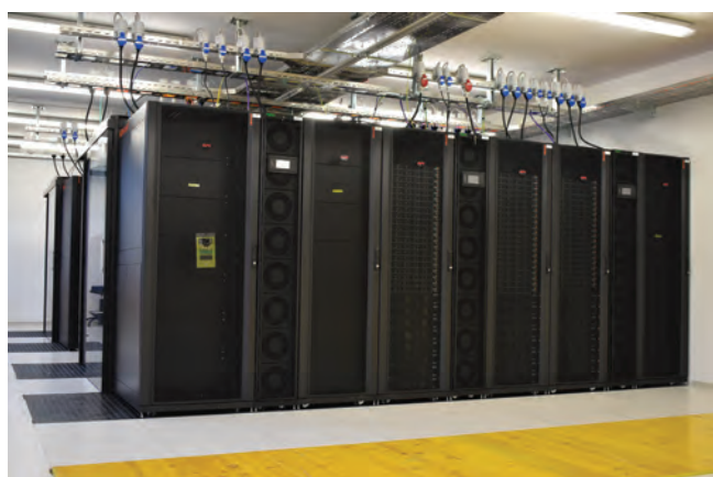
Figure 3: Additional computing cabinets and supporting infrastructure allowed for an upgrade of the NSC HPC cluster and the installation of the new Arnes HPC cluster; the most powerful public system in Slovenia at the time of installation.
