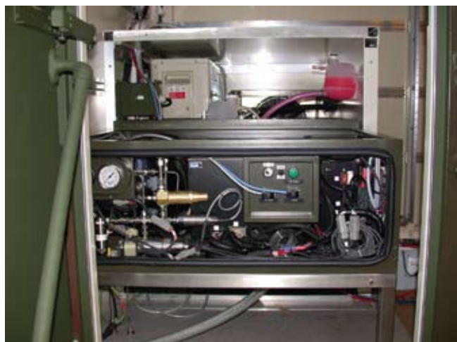
Figure 3: A 7-kilowatt fuel-cell-based auxiliary electrical power unit installed in a special purpose military vehicle
